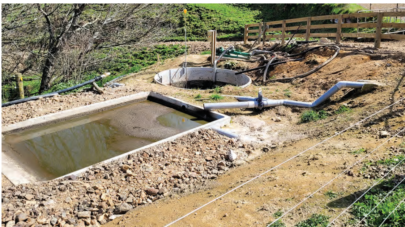
A bladder tank's stone trap sump.
